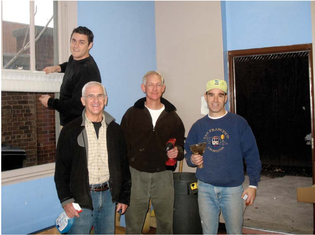
Gordon, matt, and Jim went to the Su Casa soup kitchen to repair the broken windows last winter.
